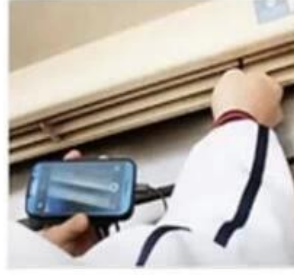
AIR CONDITIONER INSPECTION
