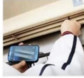
AIR CONDITIONER INSPECTION
